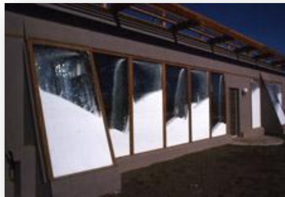
Styrofoam beads blown in between south-facing glass panes, spaced 4" apart, provide super insulation, preventing excessive heat loss during winter nights from solar gain windows.
