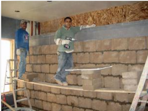
An interior adobe wall absorbs solar warmth, reduces daytime overheating, and releases heat slowly during winter nights.
